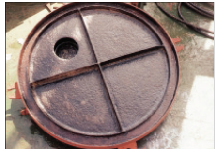
Step 6 Hatch cover surface after 3 hours application. The surface is ready for painting that must be done within 48 hours from RUST CONVERTER application.
