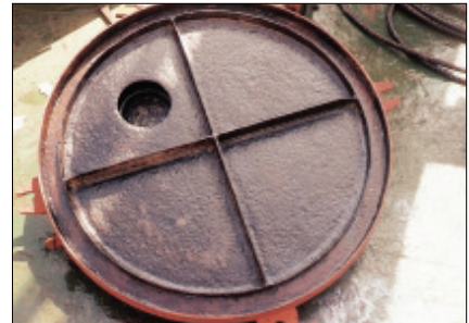
Step 6 Hatch cover surface after 3 hours application. The surface is ready for painting that must be done within 48 hours from RUST CONVERTER application.
